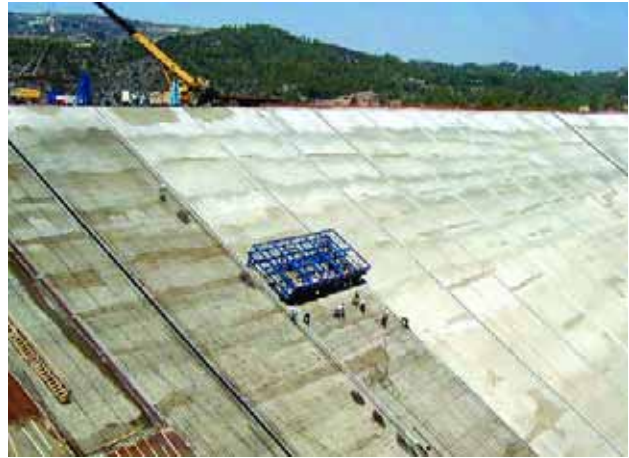
The upstream concrete face of Kannaviou dam constructed with the slipforming technique
